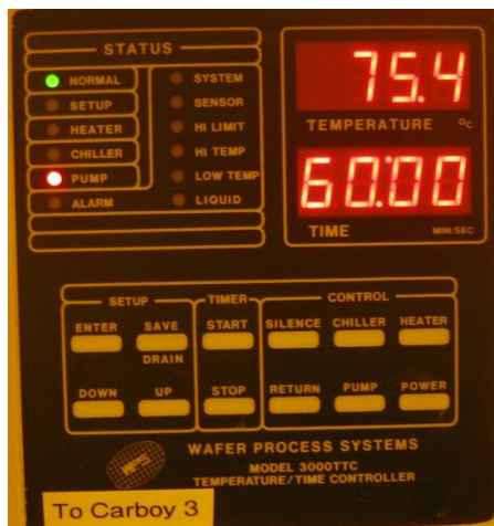
Figure 3: Control panel for KOH tank
