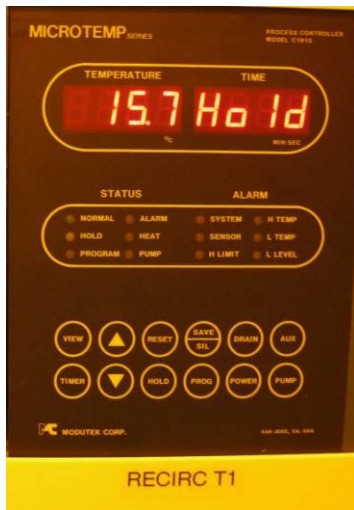
Figure 2: Control panel for RCA-1 tank.
