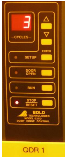
Figure 5: Control panel for QDR 1.
